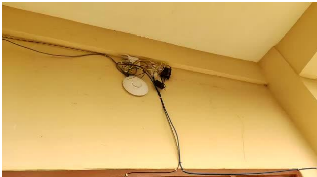
Figure 6. Evidence that the internet installation is not well maintained. (Outdoor)
