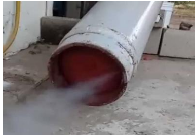
Gambar 7: Kebocoran tangki gas pabrik
